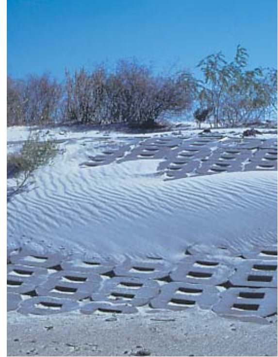
Concrete-articulated mats were installed to protect the island perimeter from tidal erosion.
